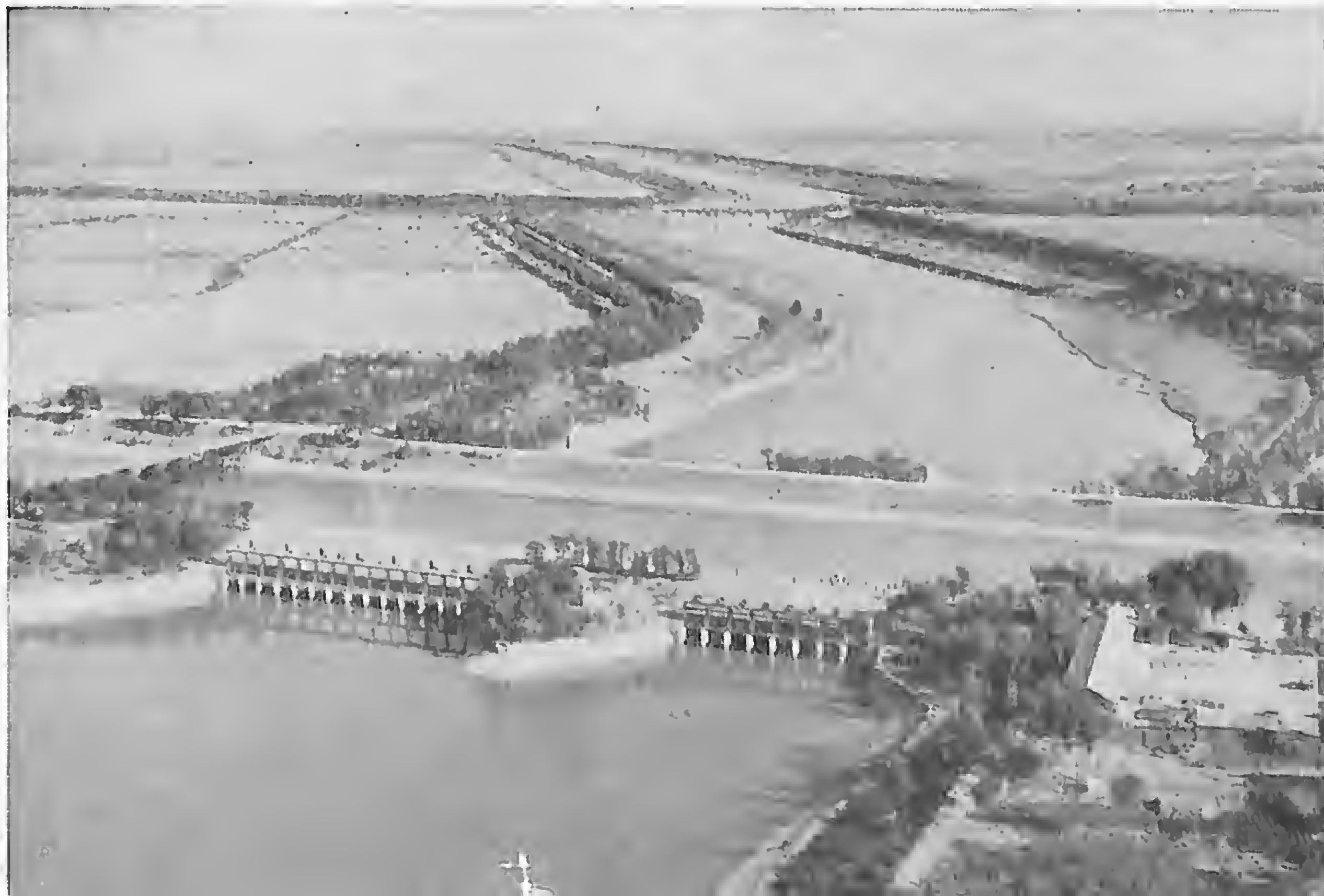
A newly completed siphon station, one of many water conservation works that control floods and waterlogging in the Haiho River basin.
